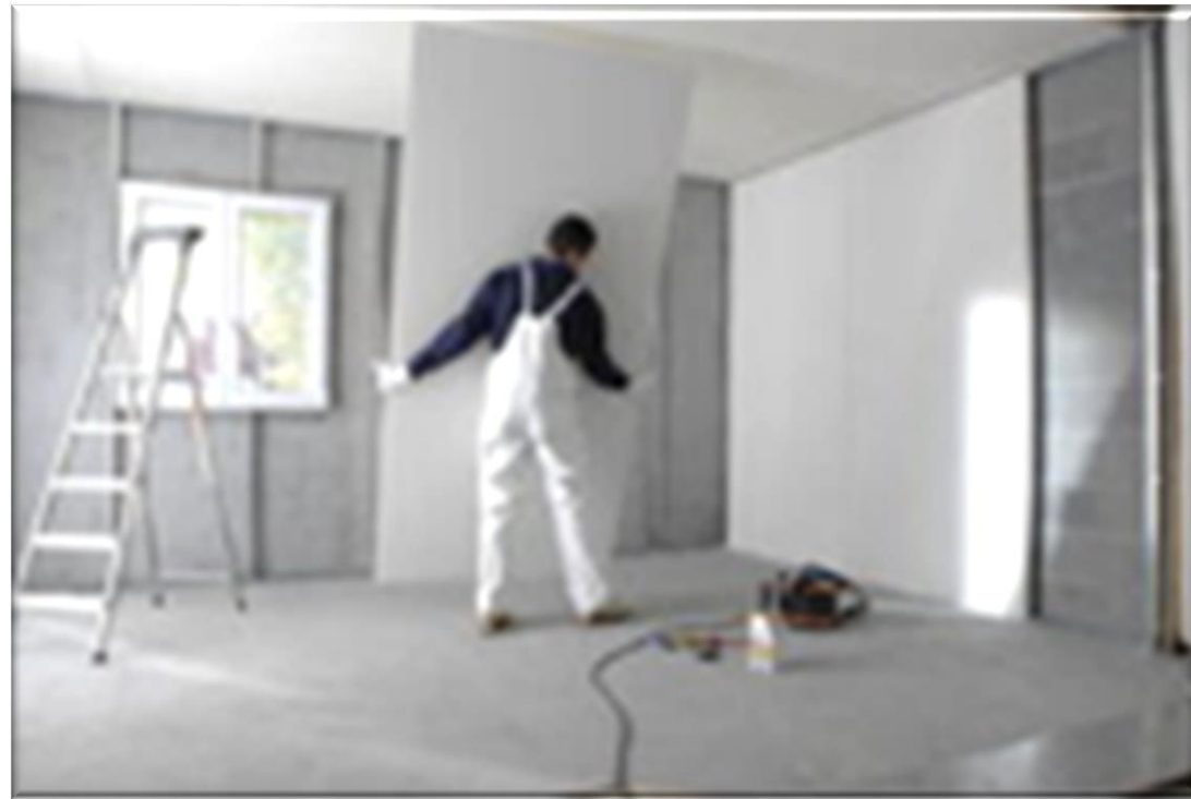
Building & Renovating in an energy and resource efficient way : light construction / building insulation
