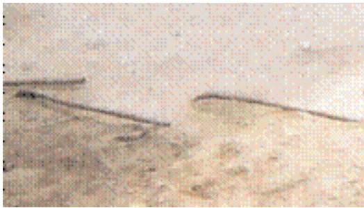
Figure 32 – Bent reinforcing steel
